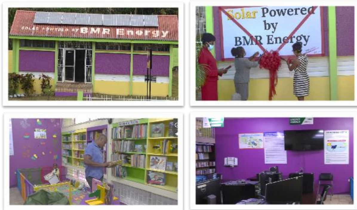
Exterior of the Malvern Branch Library –Jamaica’s first 100% solar powered public library and the cutting of the ribbon by JLS and BMR to mark the commissioning of the renewable energy system. Interior of the branch library highlighting the renewable energy corner and kiddies corner.
